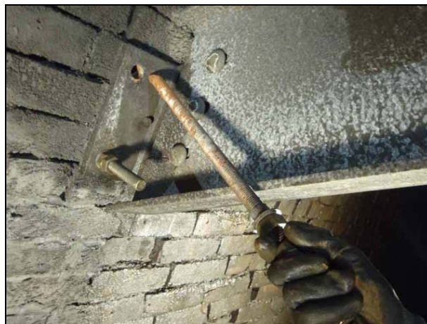
Failed polyester resin anchor bolt at Balcombe Tunnel
