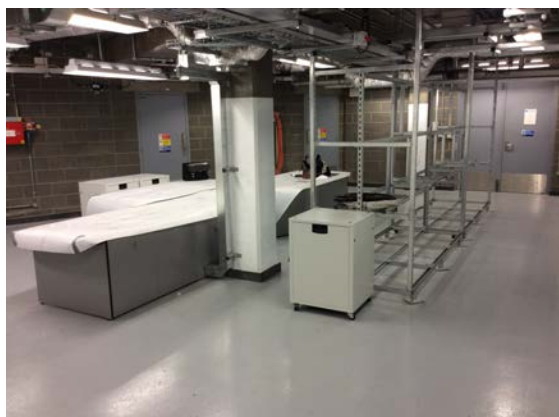
Station operations room test facility at Blackfriars
