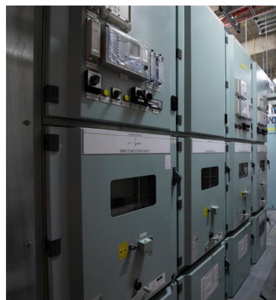
Fig. 2 Traction substation room
