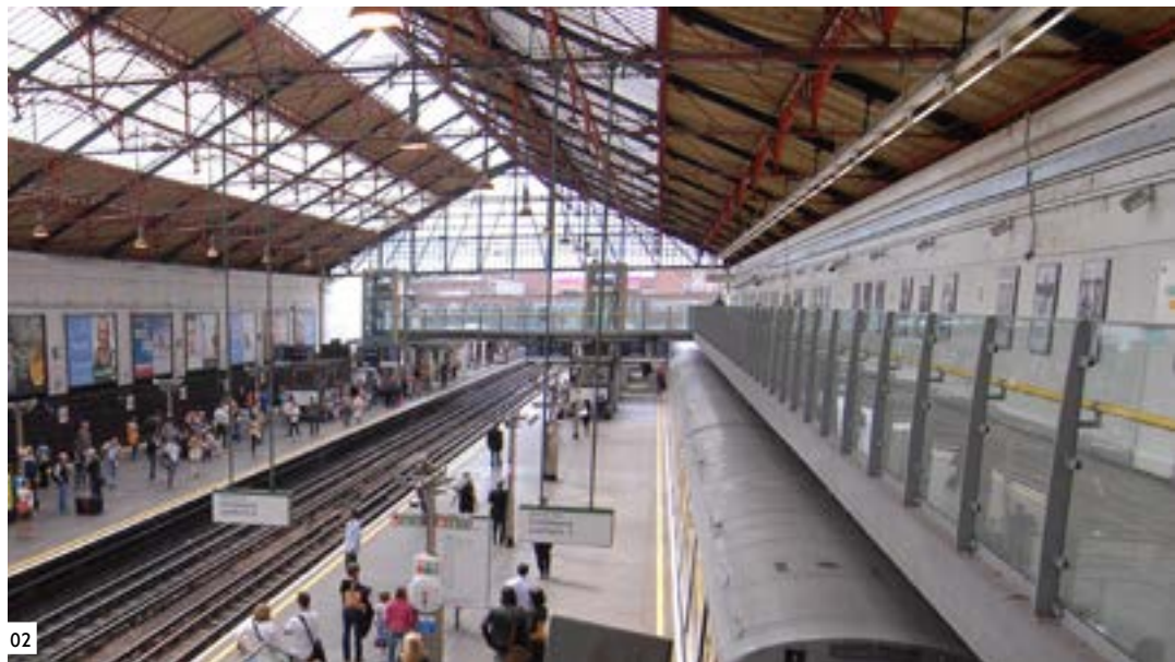
01 FARRINGDON Replacement train shed roof follows historic design but in modern materials
