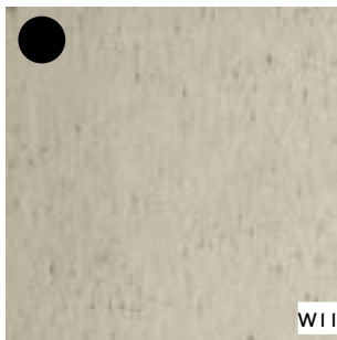
W11: Travertine stone panel fixed using proprietary cladding system with 20mm shadow gap to all sides.
