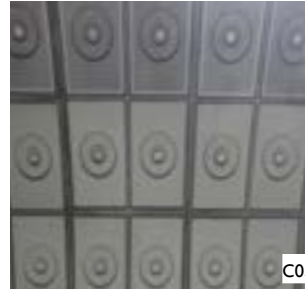
C05: Metal tunnel forming rings, dark grey/silver finish.
