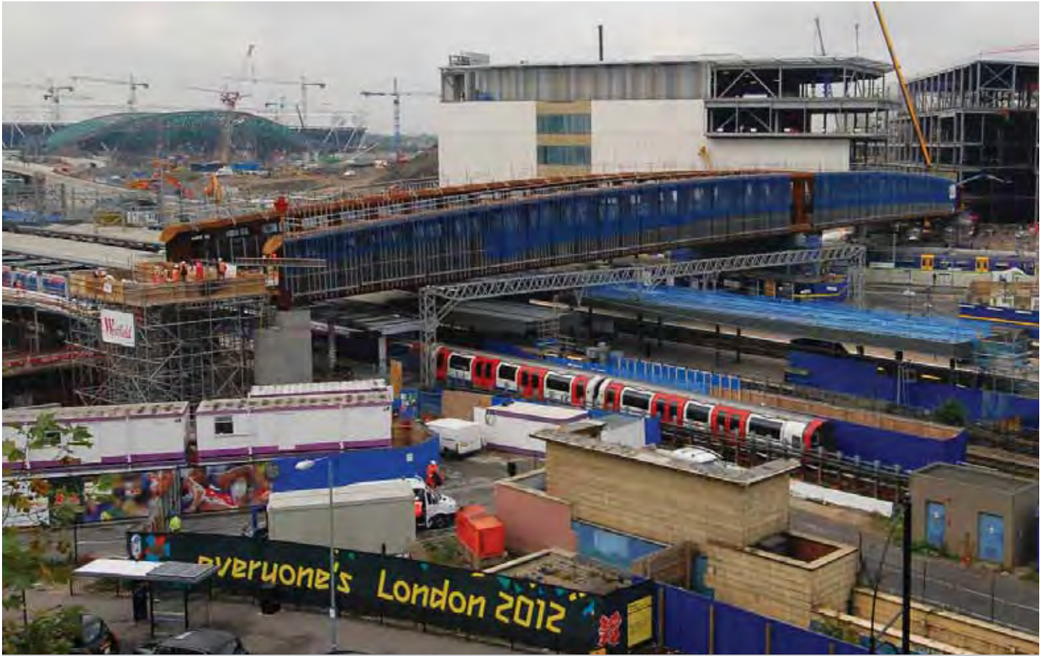
Work under way at Stratford Regional station in preparation for the 2012 Games
