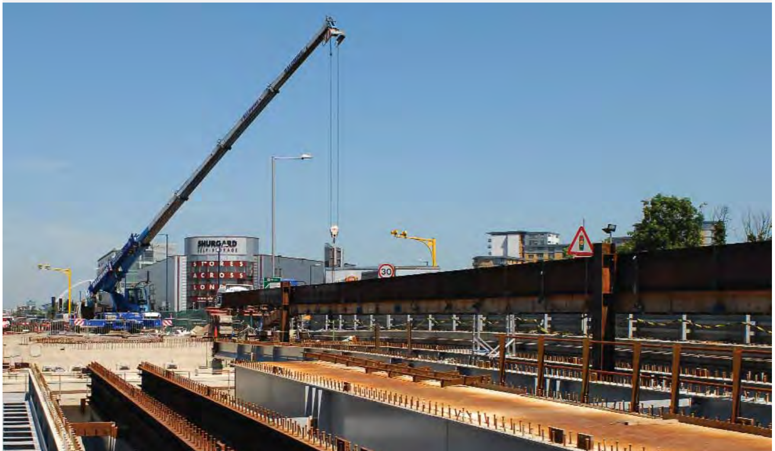
The A40 Western Avenue Bridge replacement scheme, which will create two new roads over rail bridges and secure the route over the railway for the next 120 years. It will also deliver significant improvements to cycling and walking facilities in the area
