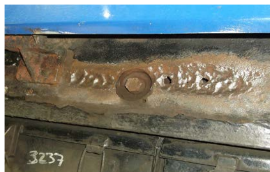
New sole bar holes and corrosion
