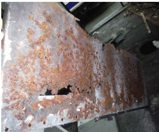
Kick plate corrosion
