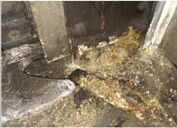
Internal door pillar corrosion
