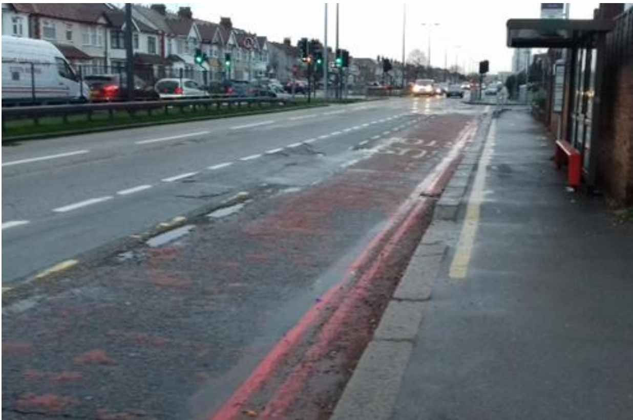
Carriageway: increasing pothole numbers (from c5,500 in 2019 to c7,200 in 2020) and poor road condition (especially at bus stops and junctions)
