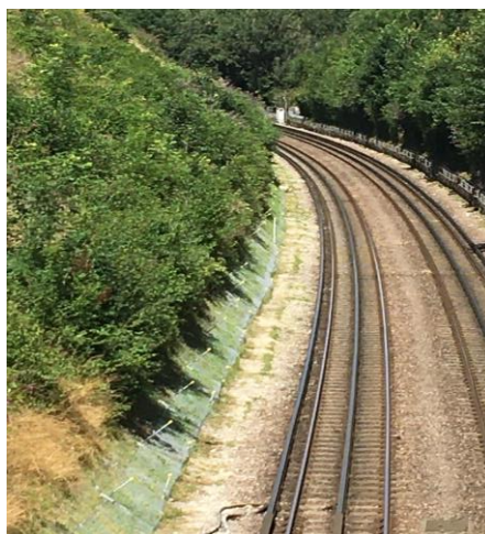
Figure 2: Stabilisation of the cutting between Chorleywood and Rickmansworth to protect the Metropolitan line train service were completed at a total cost of £4.5m
