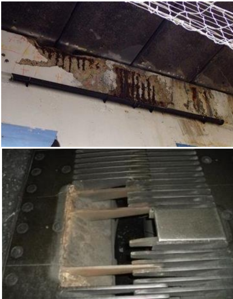
A40 Westway: Concrete deterioration and expansion joint failures; extensive works planned for 2021/22 to repair joints
