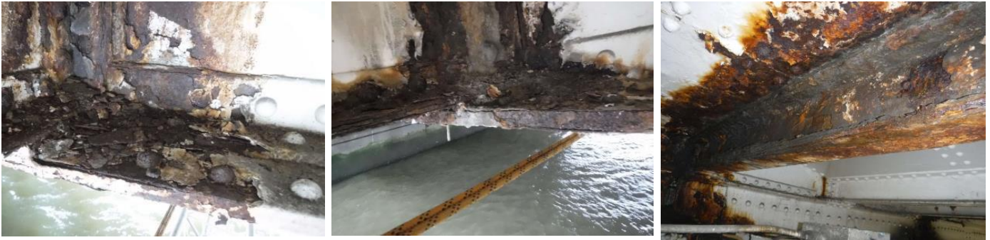
Vauxhall Bridge: Extensive corrosion on underside of bridge deck, load restriction required in next few years if this continues
