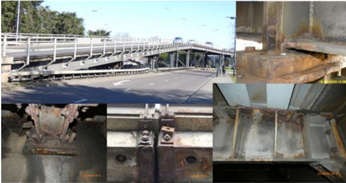
Gallows Corner: Metalwork corrosion and bolt failures requiring speed and load restrictions
