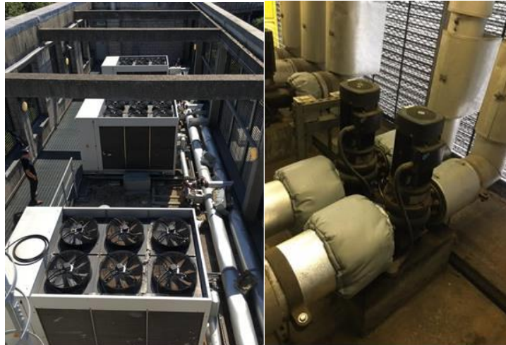
Figure 1: Works to upgrade the heating, ventilation and air conditioning system which were required to keep the Jubilee Line Service Control Centre at Neasden operational were completed at a total cost of £1.1m
