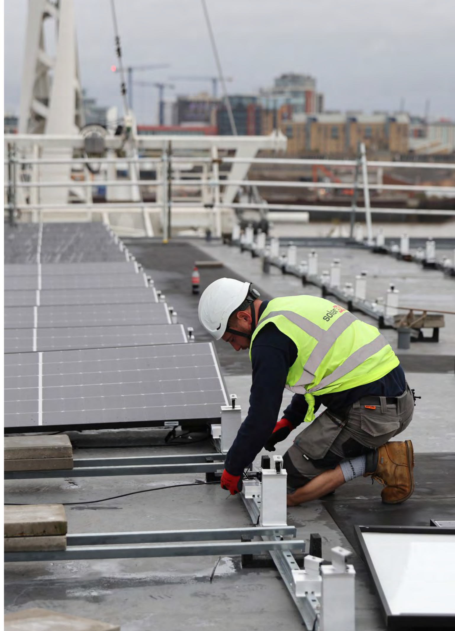
As a large power consumer, we need to make use of renewable energy
