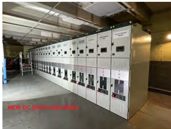
(ii) New DC Power supply Switchboards installed at Cockfosters and Northfields sub-stations
